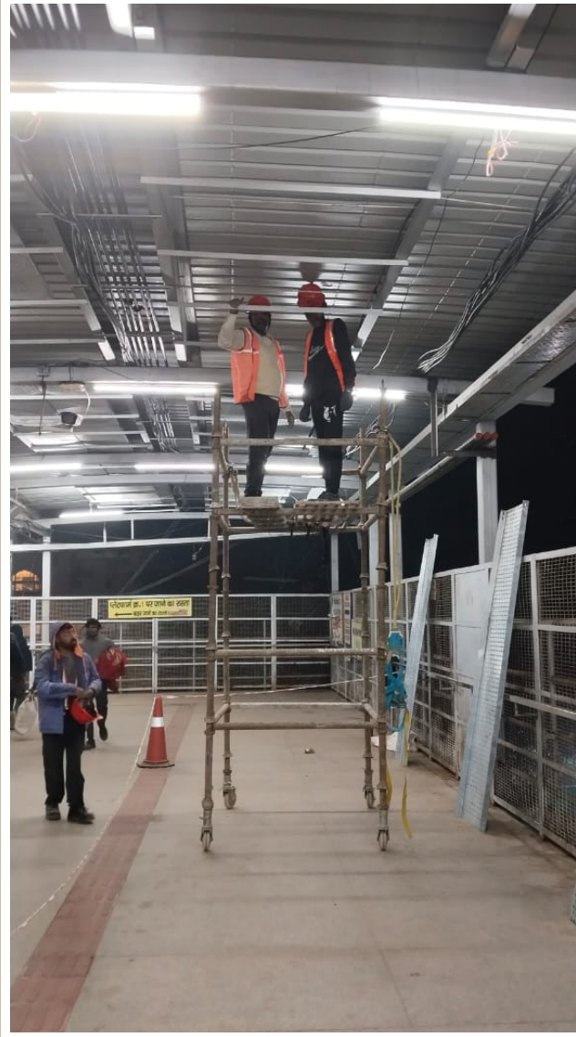
OVERHEAD CABLE-TRAY &amp; CONDUIT ELECTRICAL
