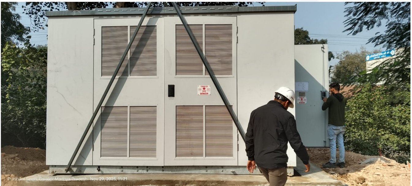
33 KV PACKAGED SUB-STATION · HT · GWALIOR
