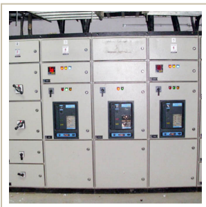
LT CONTROL PANEL
